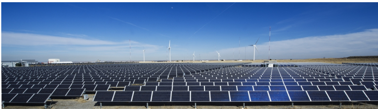
Photovoltaic panels (source: U.S. Dept. of Energy)
